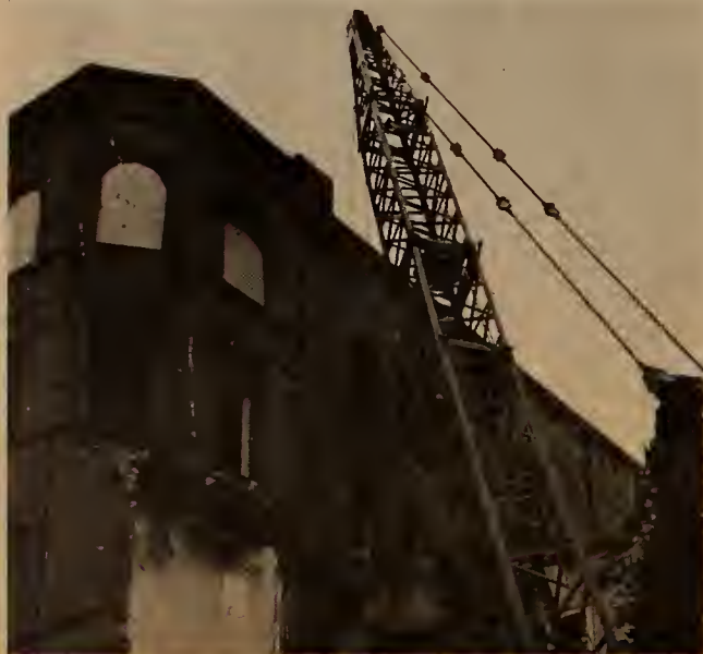
Demolition of building where the Corridor Intersects Massachusetts Avenue in the South End.
